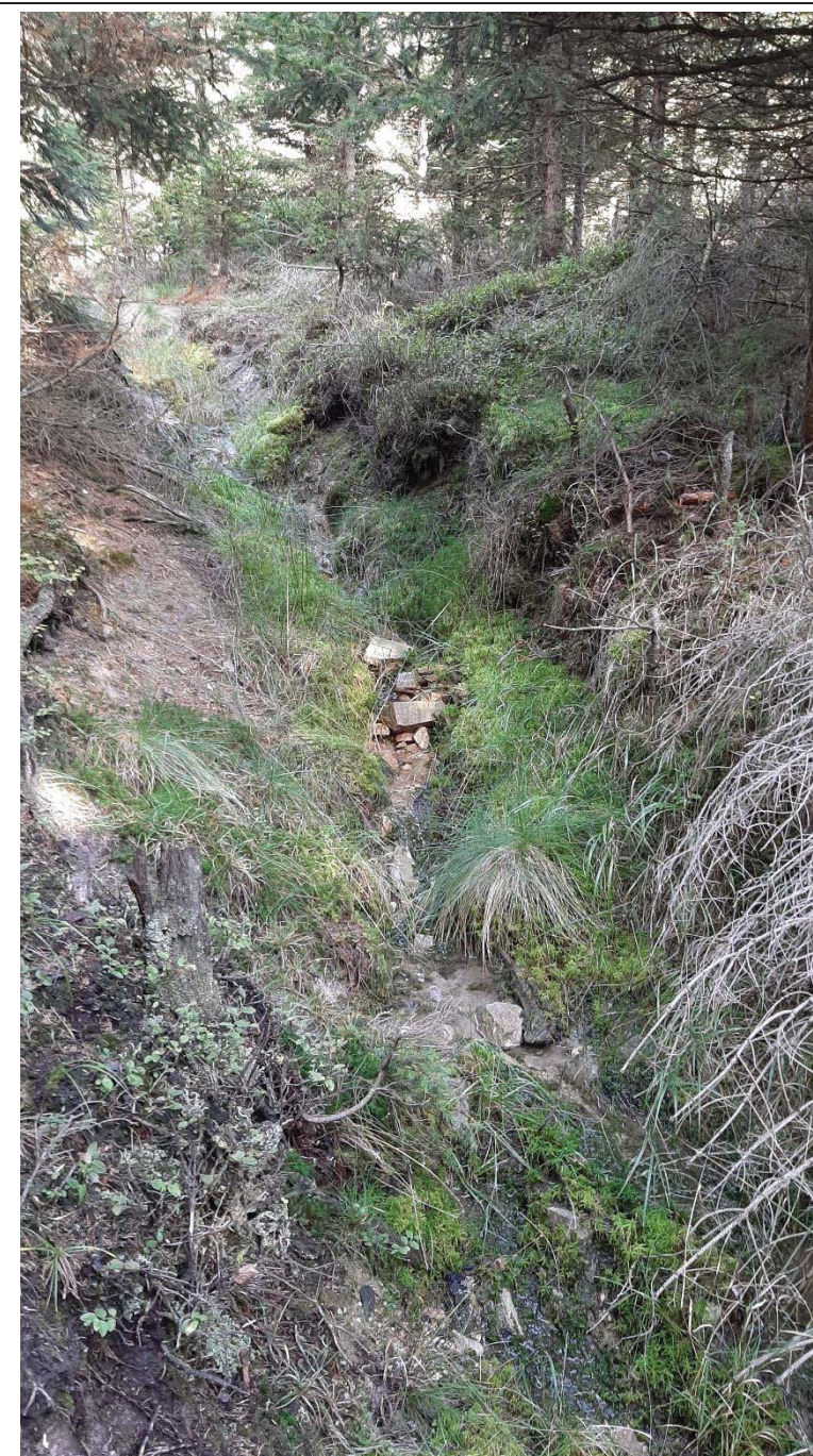
Photo 7 Depth erosion in the riverbed of a regulated small stream at site 3 Spring area of the Třítrubecký potok Brook
